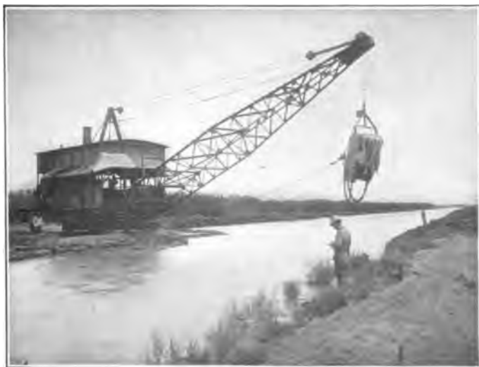
BETTERMENT OF MAIN CANAL. Enlarging by dragline while canal is in operation, in Salt River Valley, Arizona.
